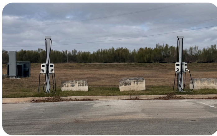
Vehicle charging infrastructure at Northeast Metropolitan Park.
