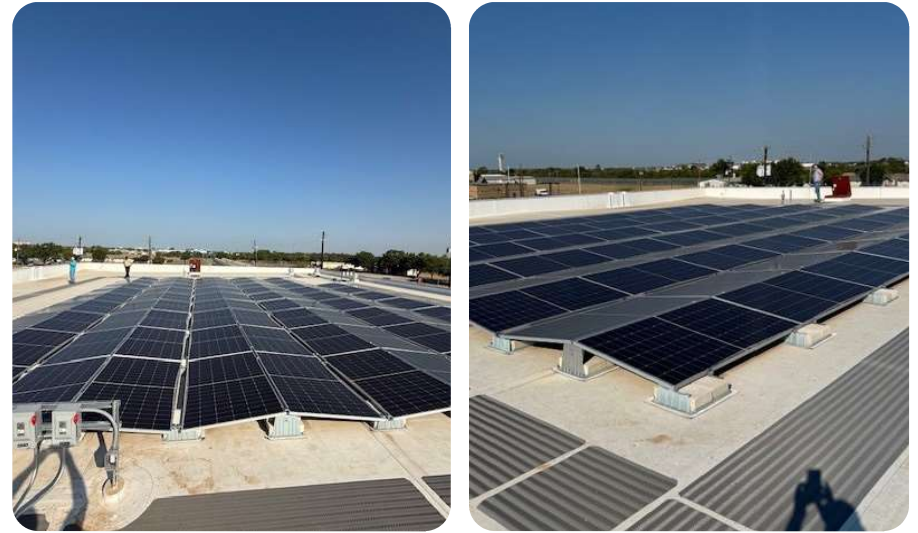
Rooftop Solar Array at the new Evidence Warehouse at the Travis County Correctional Complex.
